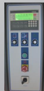
PLC controls with LED screen
